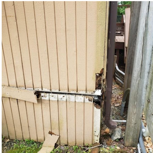
Effects of Degradation: Moisture penetration and Black Mold
