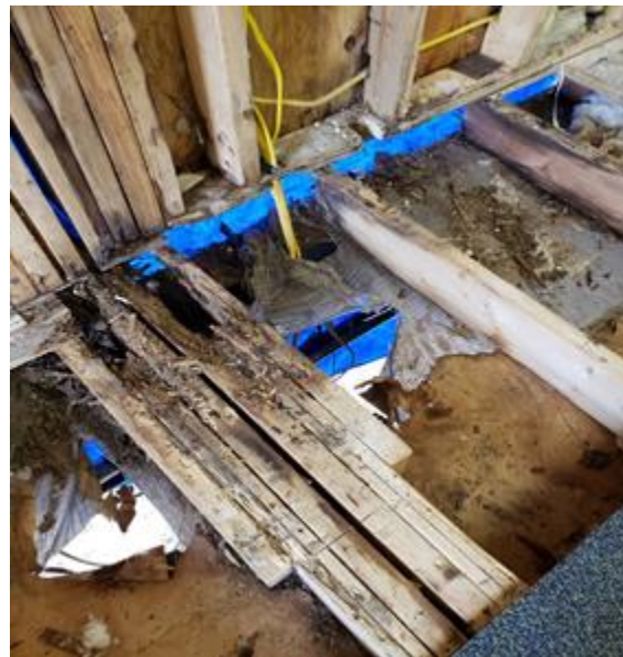
Modular Trailer: Rotting from the floor up
