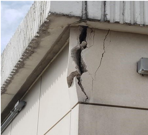
Precast Concrete Building: Structural Failure
