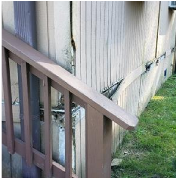
HRT Modular Trailer: Deteriorated classroom
